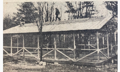
S THE NEW ARTS AND CRAFTS Northwest Hill. Workers are Harvey of Williamstown Boys' Club, located at left, and George Anderson.
